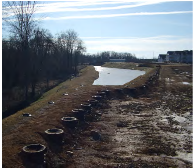
Retention Basin at Capacity after Storm
