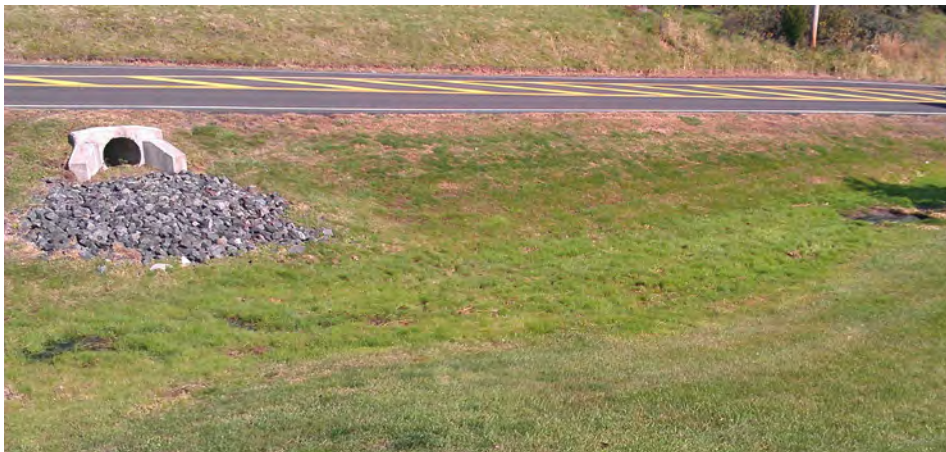
Green, but not so clean: the torn and muddy bottom of this basin suggests that it does little to slow and infiltrate stormwater and the pollutants it contains.
