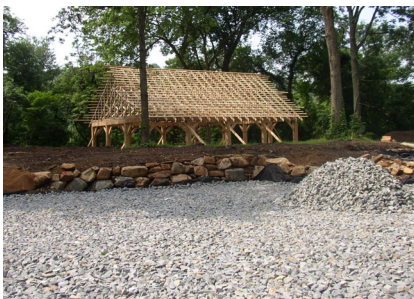
Porous paving parking lot under construction (2004). Gravel under the pavement allows water to percolate into the soil below, giving groundwater recharge.
